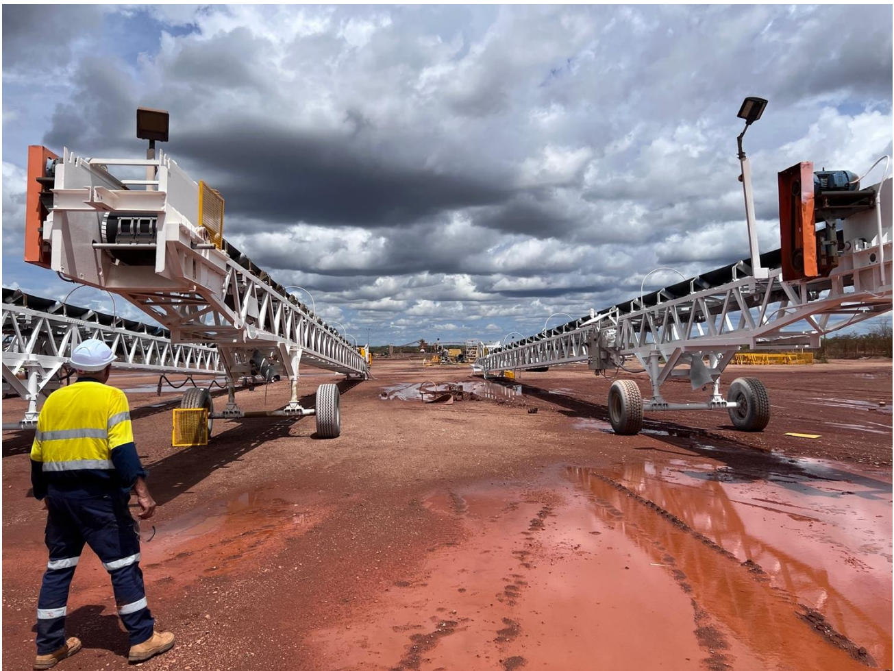
Image 8. Inspecting several of the refurbished stacking conveyors prior to reassembly and load testing.
