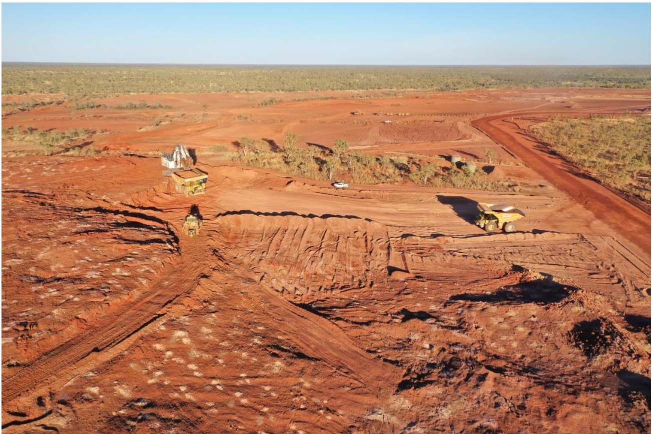
Image 9. Commencement of mining at Anthill east pit area. Clearing of pit areas, waste rock stockpile areas and topsoil stockpiles completed. Haul roads have been established.
